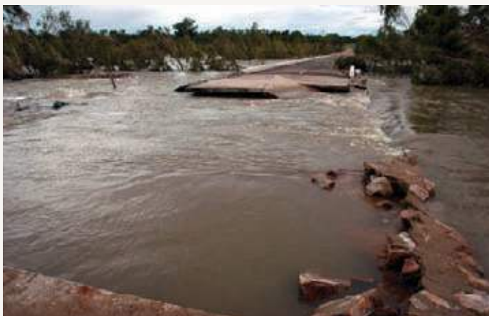
Einasleigh River, and what's left of the bridge. Repairing and upgrading this bridge to withstand future flood events is top of the list for the region's recovery plan. Photo courtesy of NGRMG.
